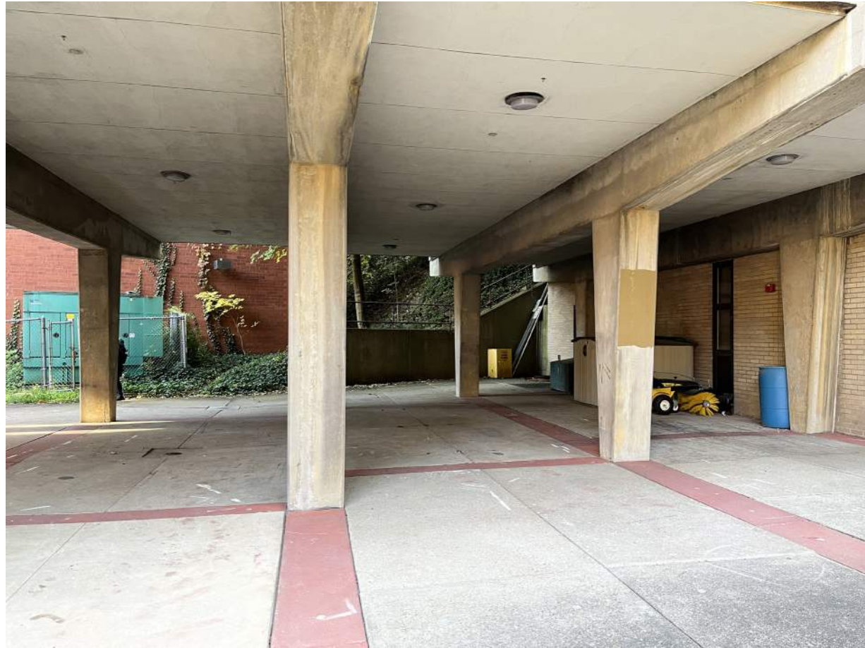
View of existing Hamerschlag House open plinth at the ground floor where new Commons will be inserted
