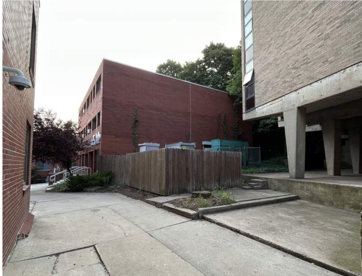
View of existing fenced area around transformer and emergency generator to be replaced with new wood plank enclosure (to match existing, but 7ft. tall to meet current electrical code).
