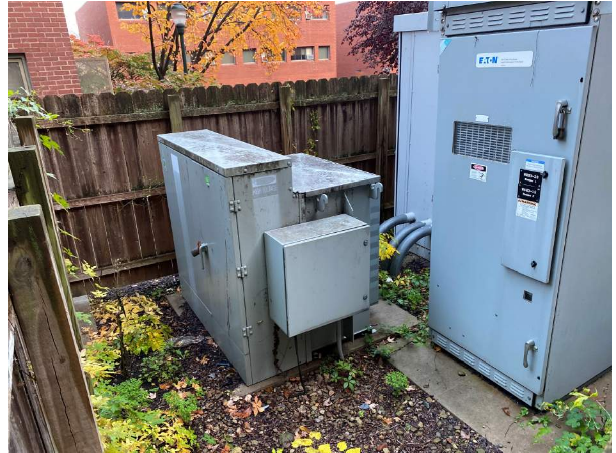
View of existing transformer and equipment to remain
